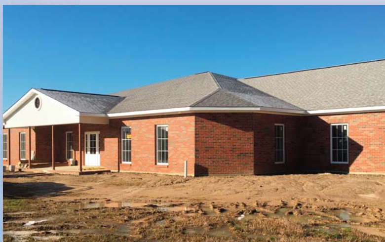
Construction on new HomePlace cottage, Irma's Place, progressing nicely. Irma's Place is scheduled to open this spring.
